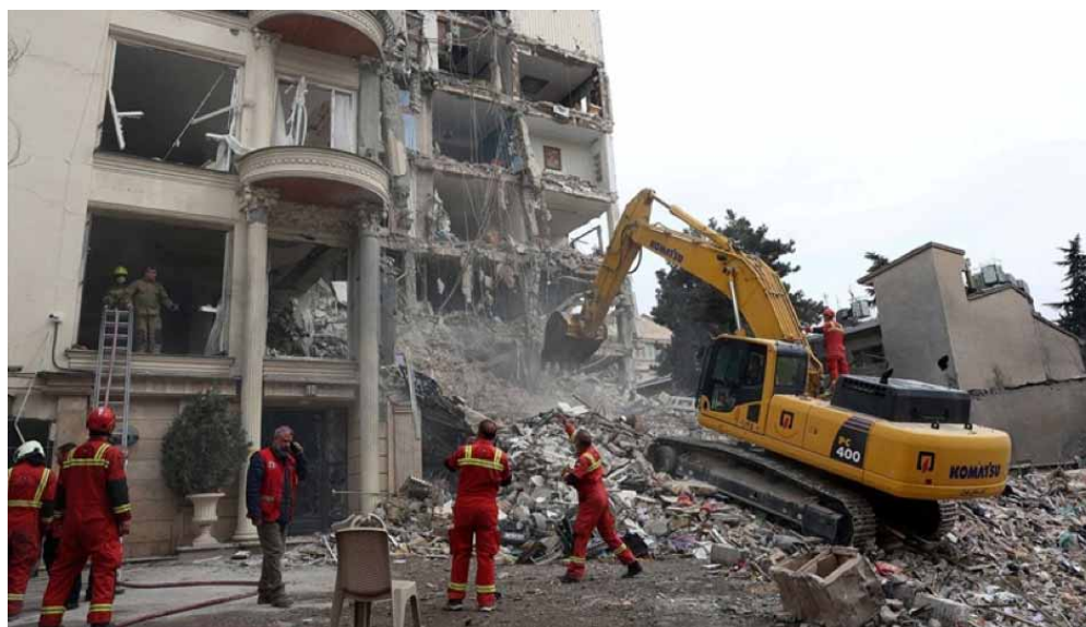
Iranian firefighters clear rubble from a destroyed residential building in northern Tehran on March 23, 2026. Photo: AFP
